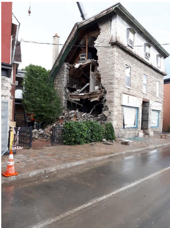
1119 Wellington Street West following collapse
