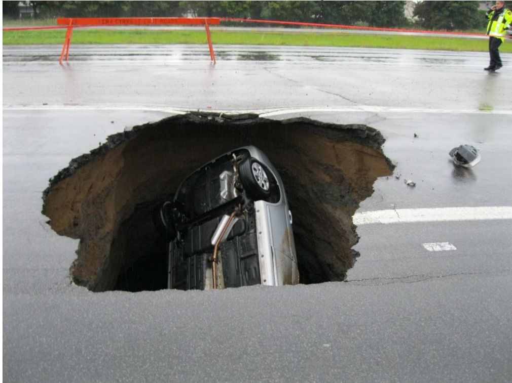
Figure 2.1 Sinkhole in Ottawa Road 174 September 4, 2012
