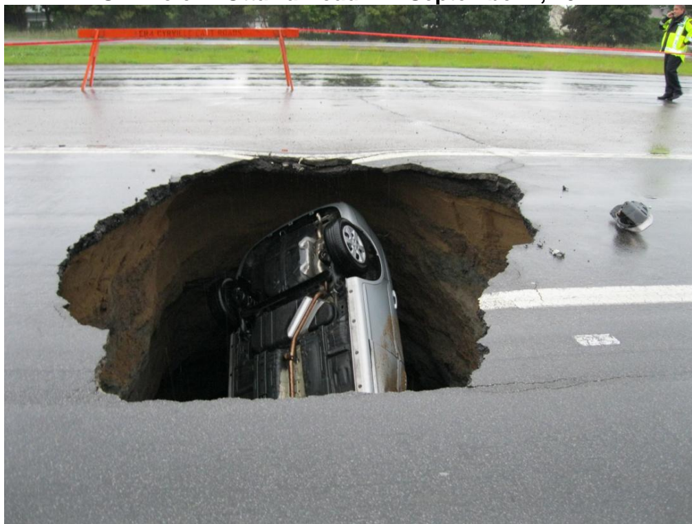
Figure 2.1 Sinkhole in Ottawa Road 174 September 4, 2012
